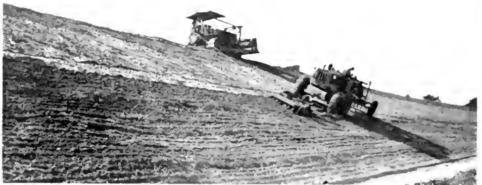
Disking 2:1 cut slope prior to spreading top soil. Grader below is cabled to tractor above
